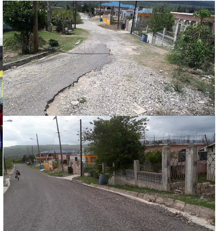
Before and after photos for the Integrated Infrastructure Project on Hope Street in York Town Clarendon
